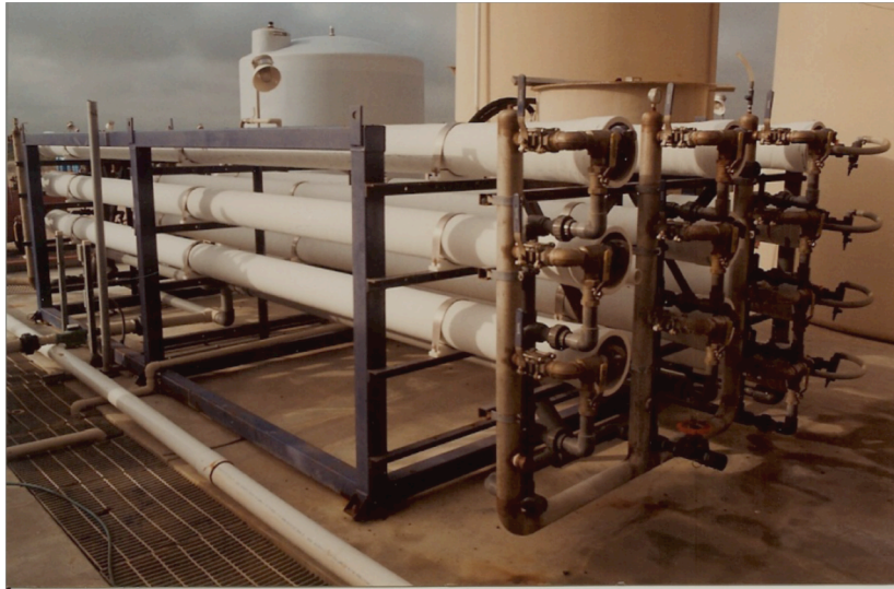
Reverse Osmosis Water Processing Equipment
